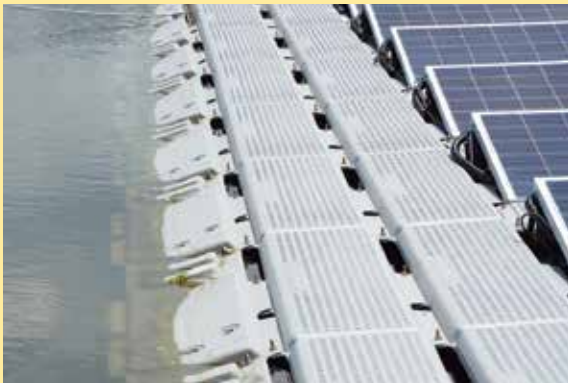
FIGURE 4.4 FPV system with semisubmerged edges used as weights
