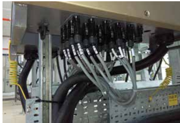
FIGURE 8.7 DC isolator switch at bottom of the inverter, and neatly terminated cables with labels
