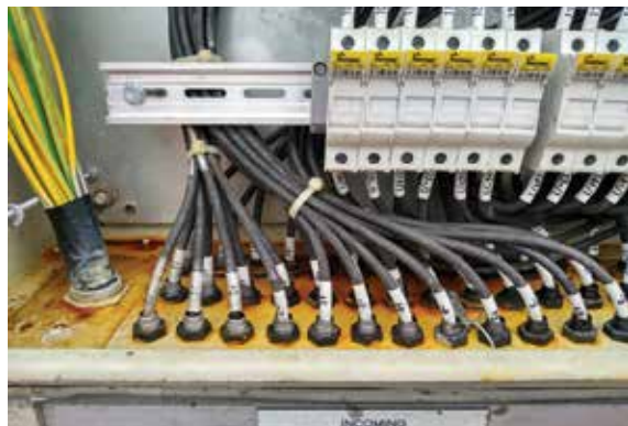
FIGURE 9.19 Water ingress and IP integrity compromised
