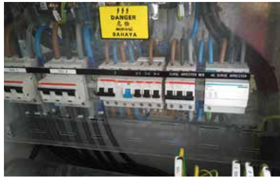
FIGURE 4.16 AC surge arresters installed on the AC electrical subsystem, Singapore Tengah Reservoir testbed
