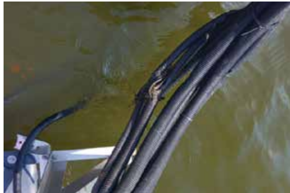
FIGURE 9.18 Conduit and cable sheath wear out
