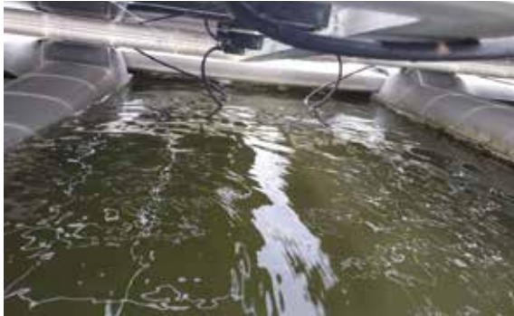
FIGURE 9.15 Connectors and cables submerged in water
