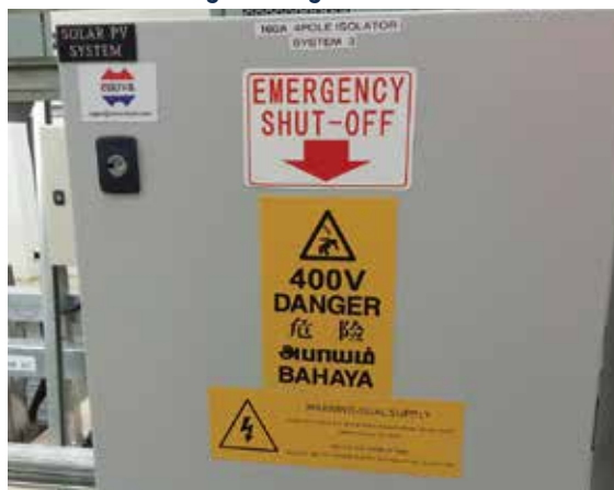
FIGURE 8.1 Safety warning labels
