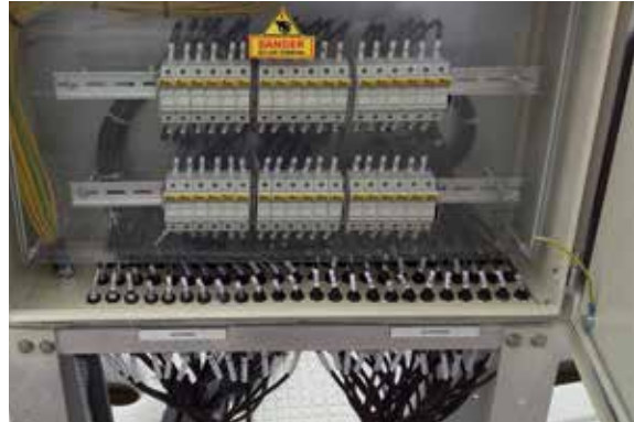
FIGURE 8.6 DC distribution board with fuses and grounding cables terminated with markings
