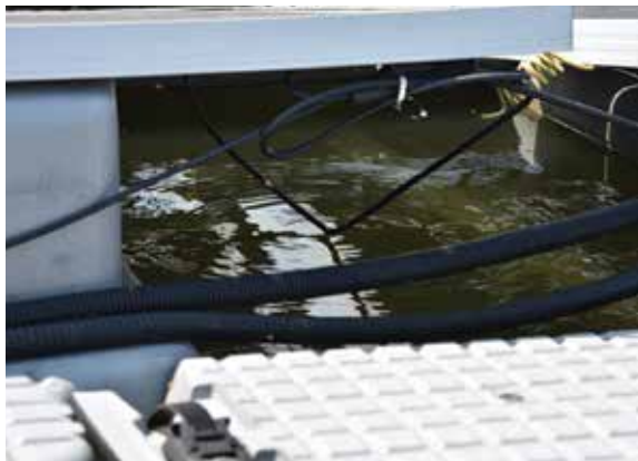
FIGURE 7.6 Examples of cables in contact with water
