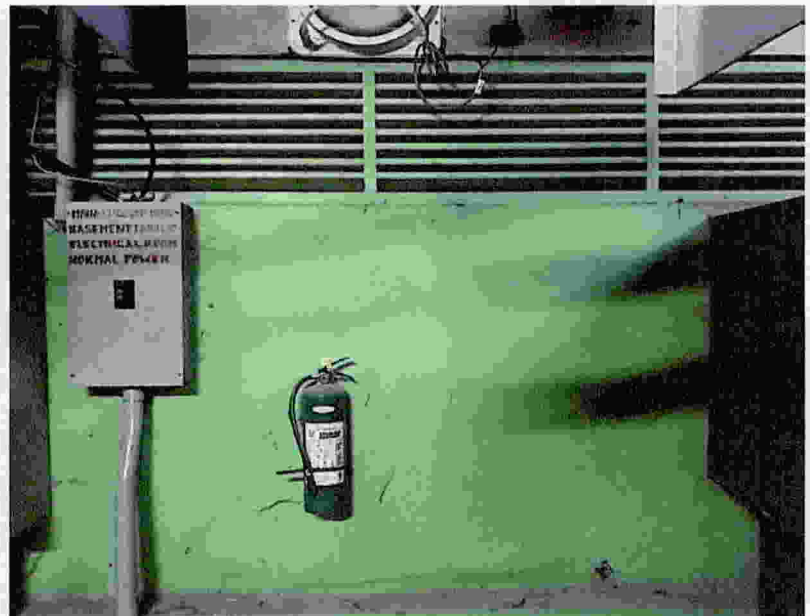
NEW LOCATION OF THE ELECTRICAL PANEL BOARDS, TRANSFORMER, & METER BASE
